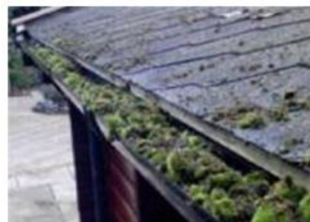
Figure 1: Unclean gutter a threat for the roof construction (JT Gutter Cleaning, 2013)
