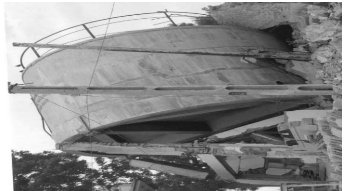
Figure1: Failure of elevated water tank in bhuj earthquake in Bhachau.
