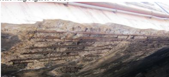
Figure.1(a) Corrosion Effect of Alluri Sitaramaraju Bridge
