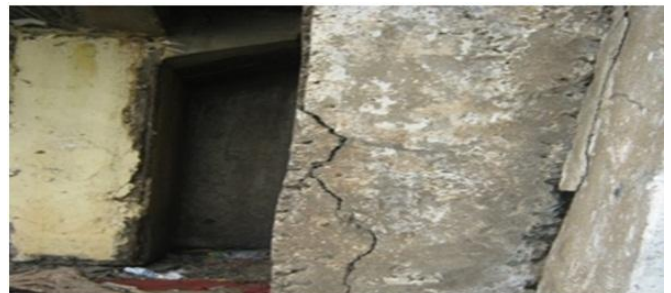
Figure 3. Cracking Effects of Eluru Locks
