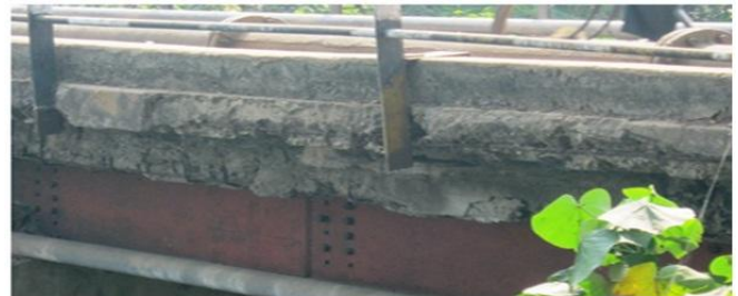
Figure 2. Picture showing signs of the Spalling of the bridge at Gunadala
