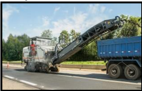
Fig 2 Efficient milling and granulating of road pavements Cold milling machines are utilized for the snappy, very proficient evacuation of black-top and solid asphalts. In doing as such, they make an even, consistent with profile base for the construction of new surface courses of uniform layer thickness. What's more, milling individual asphalt layers empowers the material to be recovered in a particular procedure and isolated into the distinctive blend sorts.
