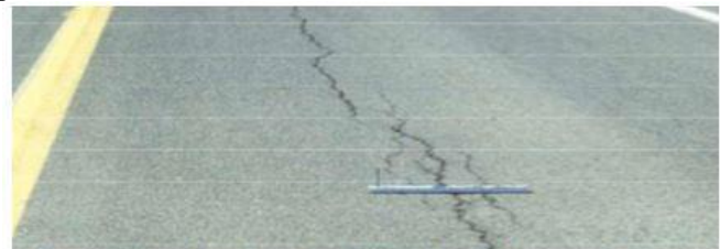
Figure 2.6: Longitudinal Cracking (Medium Severity)
