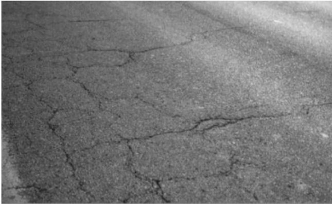
Figure 2.3: Longitudinal Cracking (Medium Severity)
