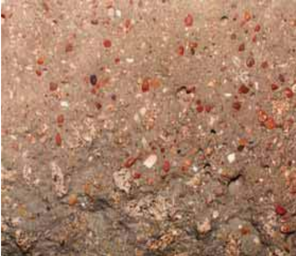
Fig: Color change in the concrete due to elevated temperature
