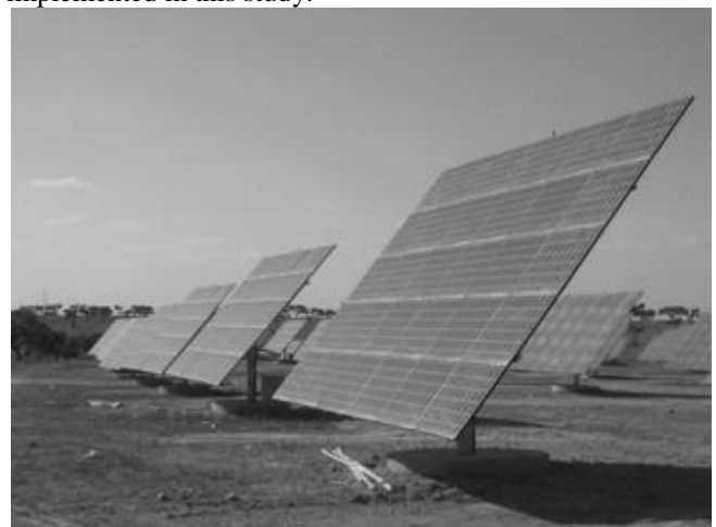
Fig. 4. Solar Park – PV panels
