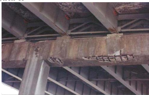
Figure 1. 1 Corrosion of a cross girder that supports the main bridge deck
