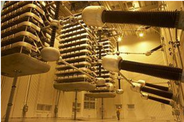
Fig.3. Thyristor valve stacks for Pole 2 of the HVDC Inter-Island between the North and South Islands of New Zealand. The man at the bottom gives scale to the size of the valves.
