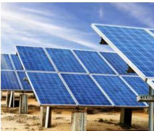
Fig 2. Solar PV System
