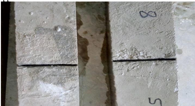
Figure 6 creation of crack
