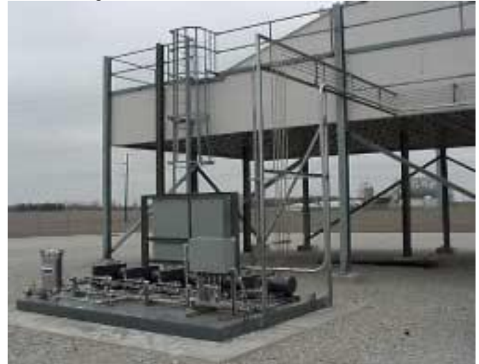
Figure 2. Typical high pressure fogging skid. The feed lines from the high pressure pumps to the inlet system can be seen here.
