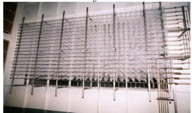
Figure 3. High pressure fogging skid in operation for a heavy-duty gas turbine.
