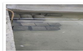
Figure-11 Water Tank
