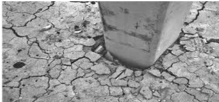
Figure: 4- Sulfate Attack
