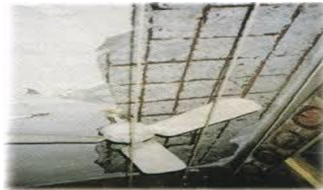
Figure: 1- Corrosion induced cracking
